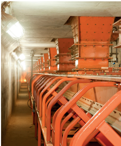
Belt Conveyor for unloading warehouses (54")
