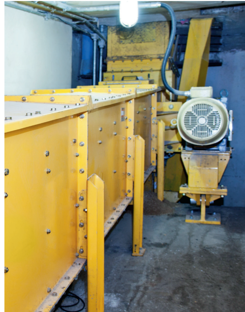
TCRA for unloading the hopper
